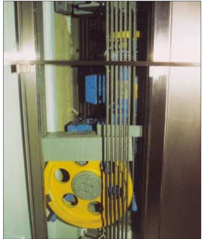
Flender elevator drive for rated load Q = 825 kg and cab speed 1 m/s. Roping ratio 2:1 Loher lift motor LUGA-132LN-04, 7.5 kW RUPEX coupling type RWB, size 125 Double shoe brake for T_{\text{brake}} = 2 \times 80 Nm Worm-helical gear unit CG26-100, ratio = 18.75 Traction sheave dia. 450
